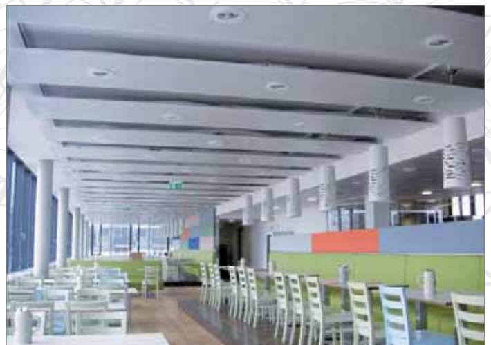
Acoustic ceiling islands in a cafeteria (Munich)
