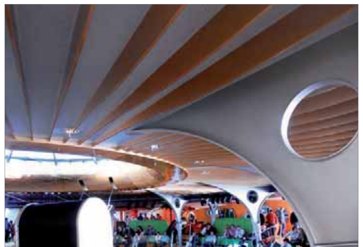
Perforated ceiling panels in a cruise liner (Aida)
